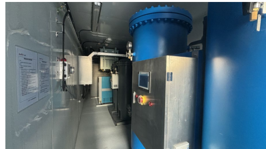
Life support system – Oxygen plant (Suhai No. 1)
