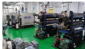
Slurry Ice Plant
